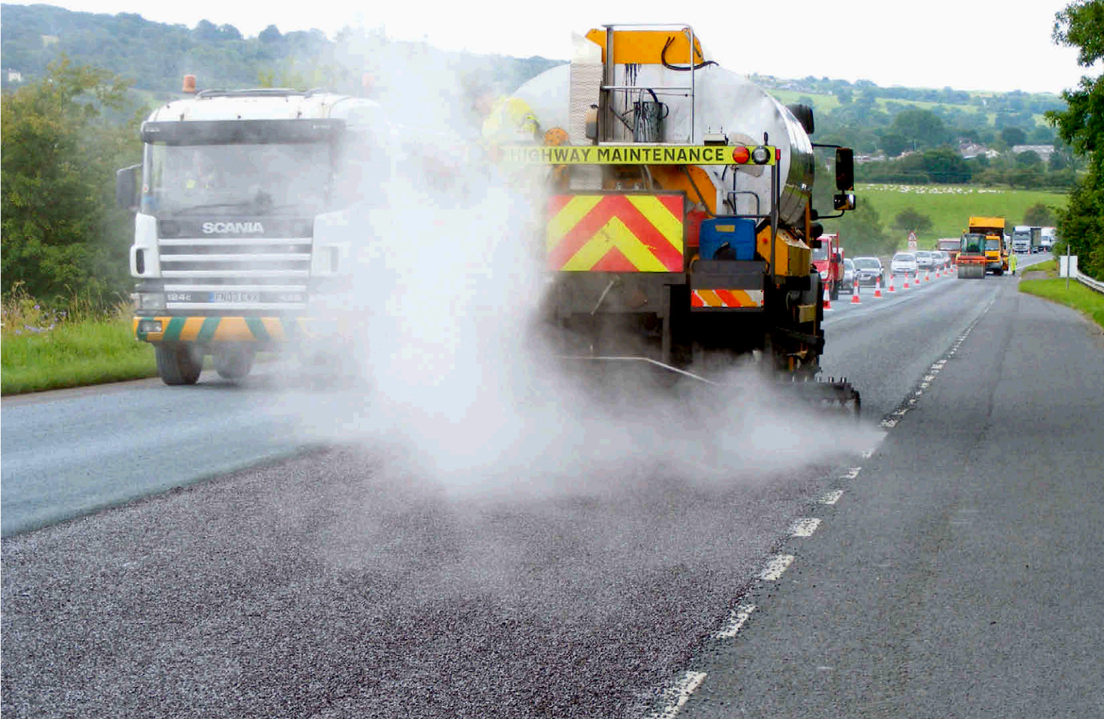
Surface dressing can restore skid resistance and inhibit the formation of potholes before more expensive repair work is required
