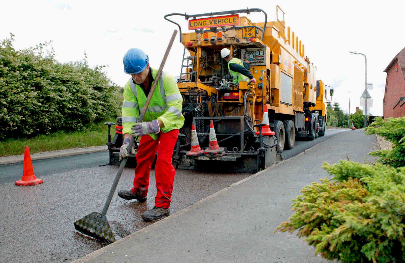
Surface treatments are growing in popularity among local authority clients with limited funds
