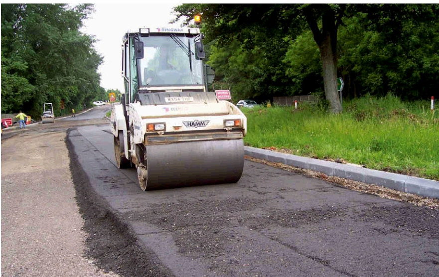
Rolling the recycled asphalt is a key part of the Foambase process
