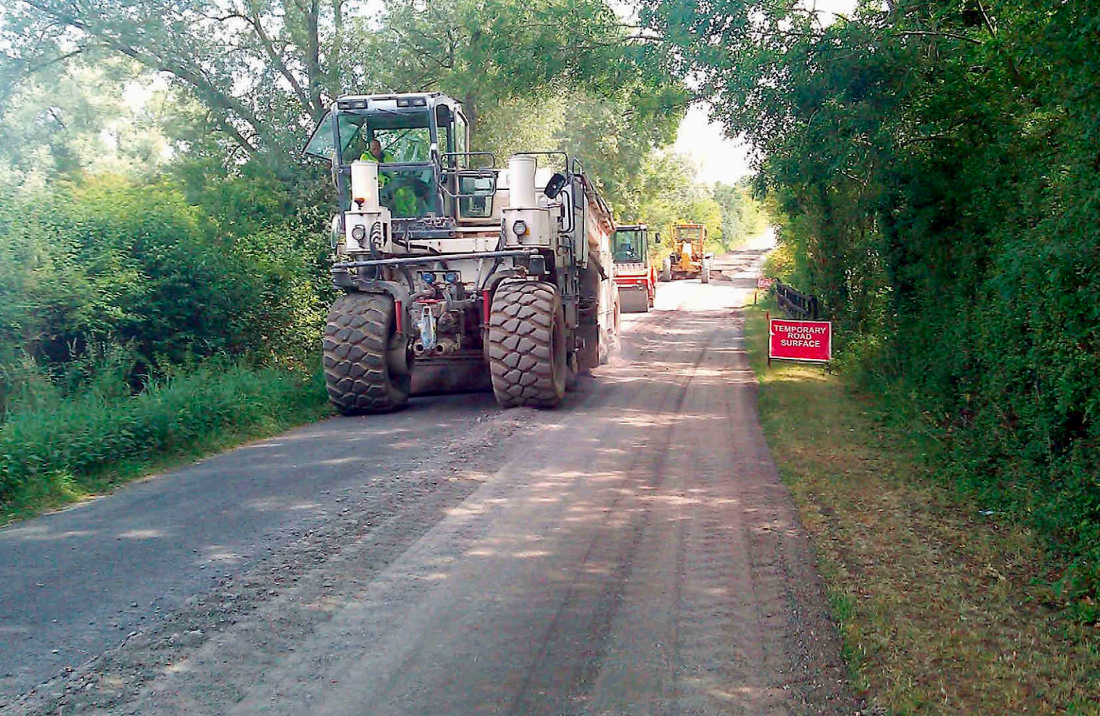
Tarmacadam that has been down for many decades is more likely to contain hazardous materials
