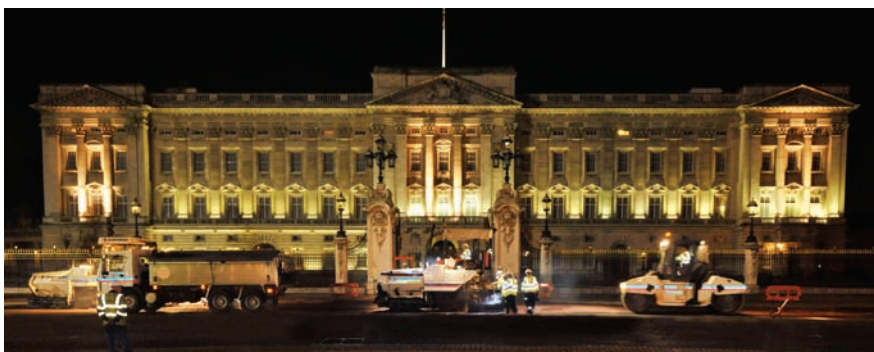
Eurovia's night work allowed tourists to view Buckingham Palace unobstructed by surfacing operations
