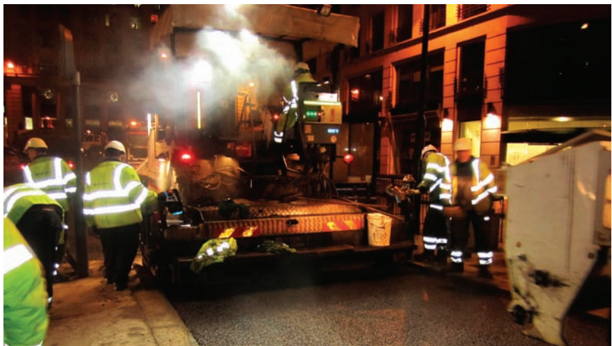
An initial pilot project of TfL's long life pavement initiative has been carried out near Monument Station
