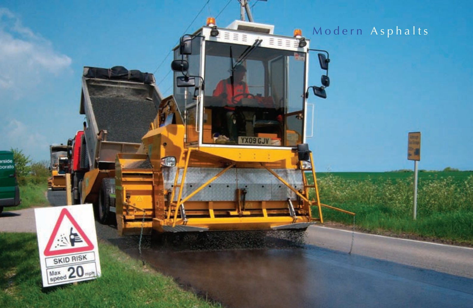
Programmes of surface dressing making use of premium binders have been specified by East Riding's Streetscene Services
