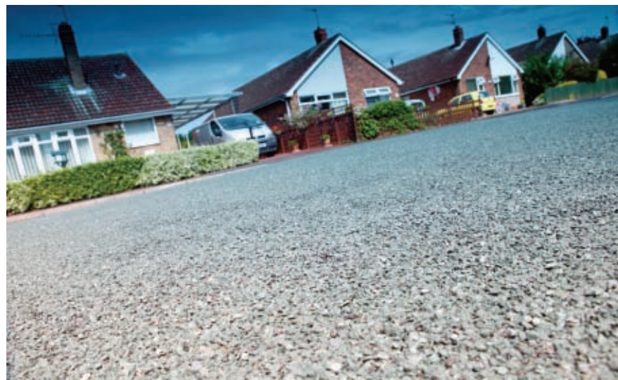
Demand for surface dressing techniques with inherent strength is likely to increase due to pressures on budgets
