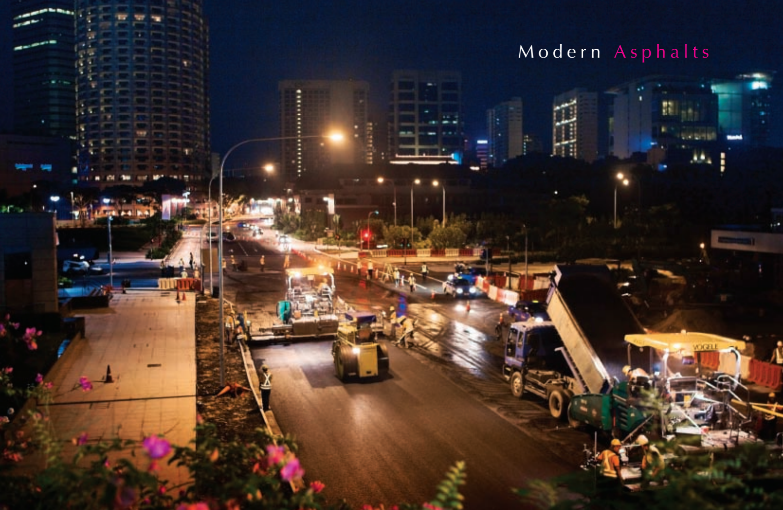
Asphalt containing Shell Cariphalte Racetrack was laid in Singapore on roads used for the city's first Formula 1 Grands Prix in 2008
