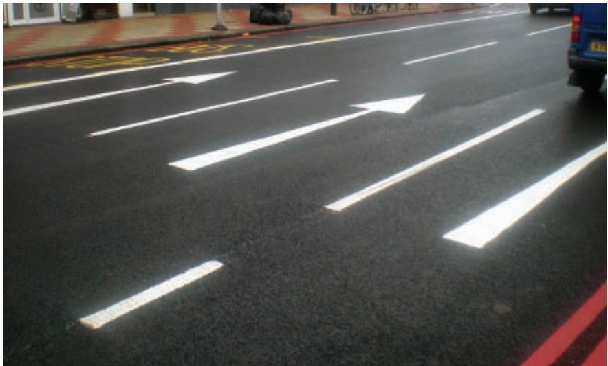
The A24 London Road has been resurfaced with a high quality asphalt in Morden
