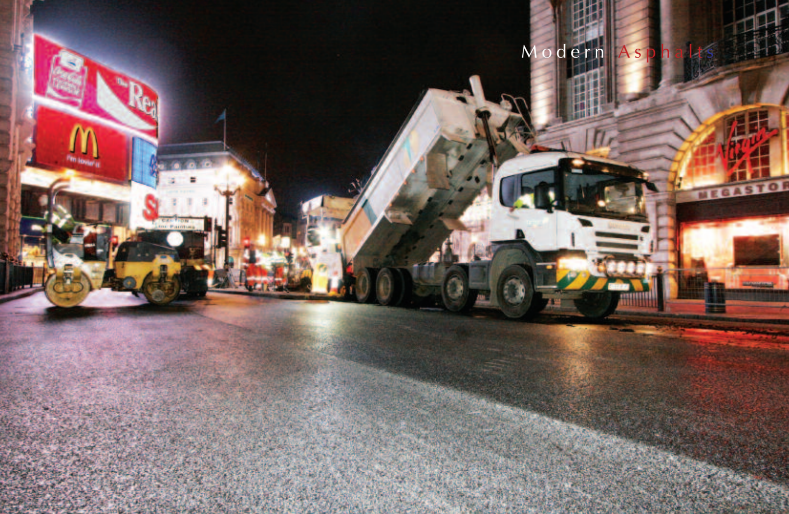
Tarmac National Contracting laid bespoke high performance asphalt in Regent Street (above), Oxford Street and Oxford Circus successively over 12 nights
