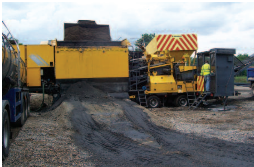
Ringway established its recycling plant beside the A338 site, saving a huge number of lorry movements
