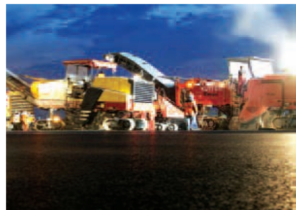
Use of Shell S-Grade binders made it possible to reconstruct the runway to its full depth each night
