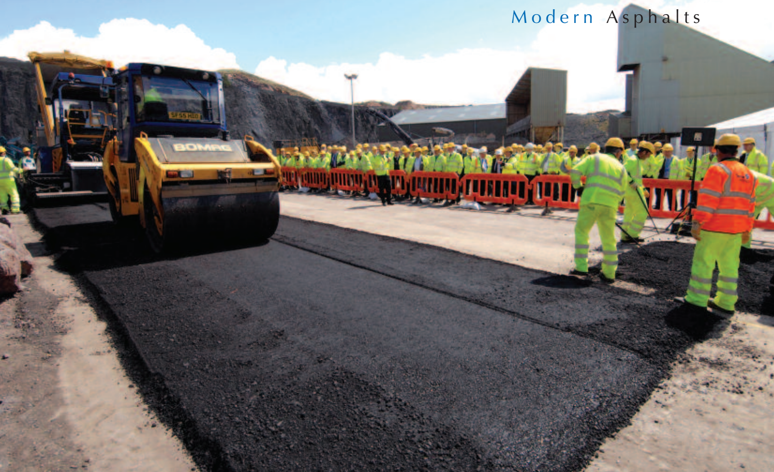
An enthusiastic group of politicians, road authority engineers and contractors watched the Tayset demonstration
