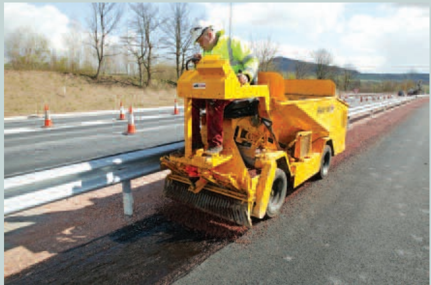
Colas' specially developed small plant was used to apply Fibredec along the central reserve strips
