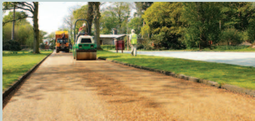
Reconstruction with Fibredec has produced a strong and aesthetic entrance to Tatton Park
