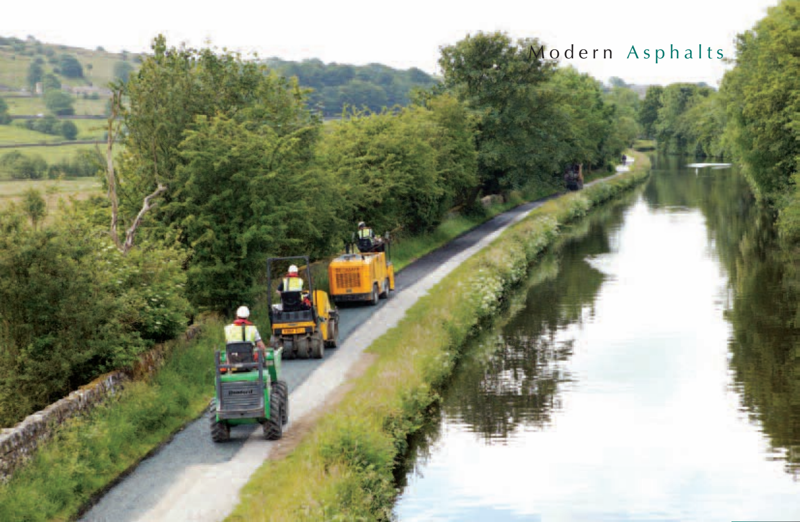
Colas has recently developed bespoke plant for laying Fibredec in tight and access restricted locations such as towpaths
