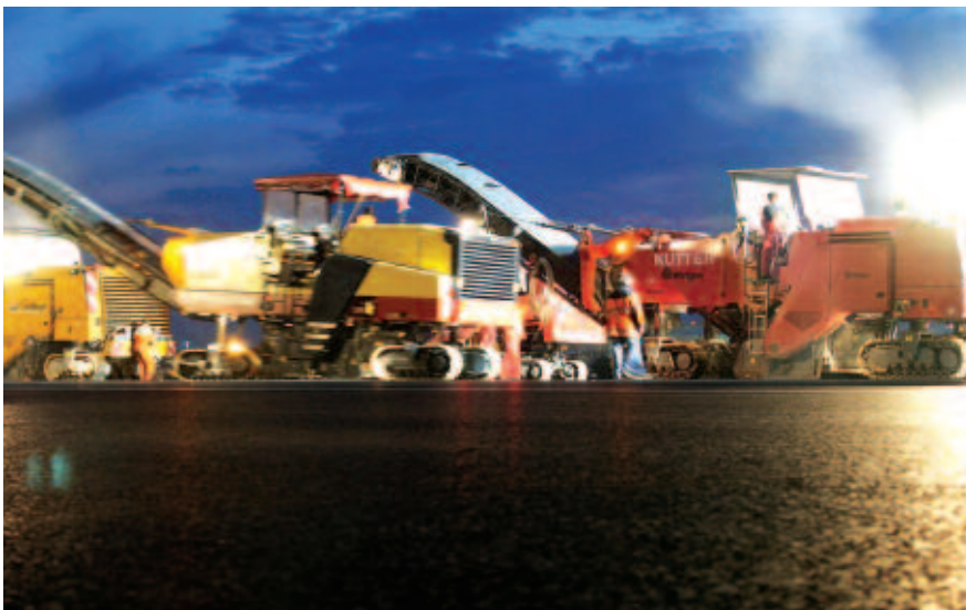
The top 40mm of temporary surface at Frankfurt was planed off and replaced with a high performance S Grade surface course at intervals of every eighth strip
