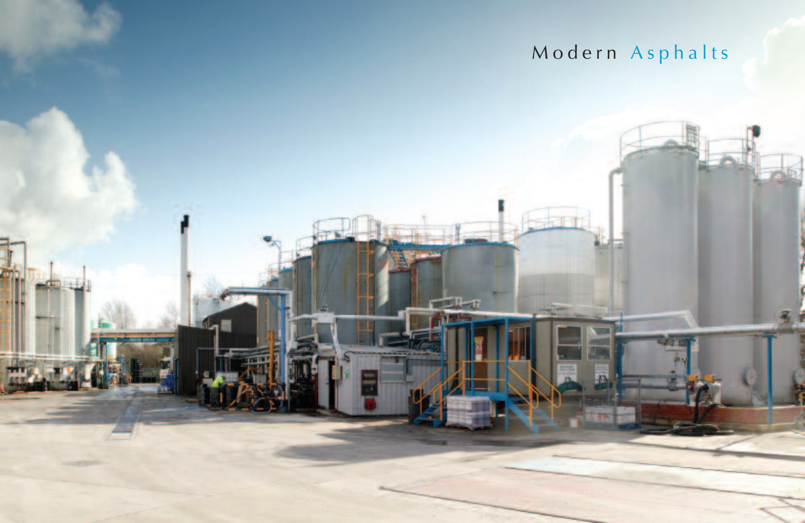
Colas' bitumen emulsion plant in Warrington. "Our asset," says Colas Business Manager for products Sommerville Wright
