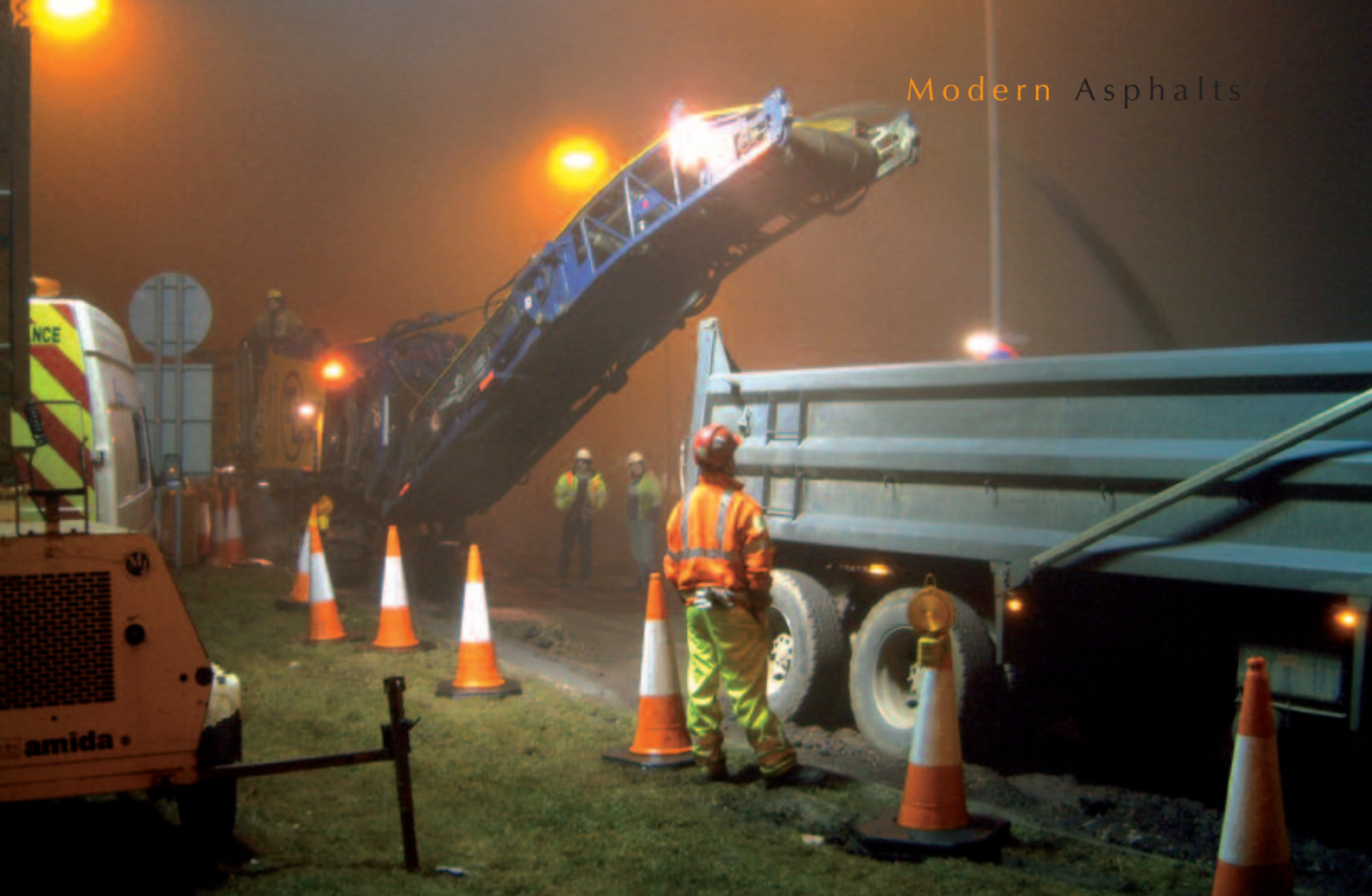
Planings from the A46 were recycled using Viafoam and relaid as a base course over the crack and seat treated concrete sub base
