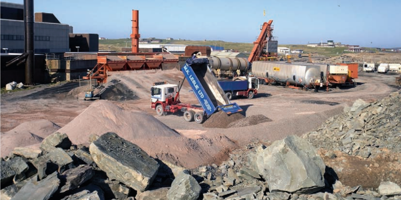
Colas took the UK's largest mobile asphalt plant to the Shetland Islands to produce up to 200t of BBA asphalt per hour for surfacing Sumburgh's main runway
