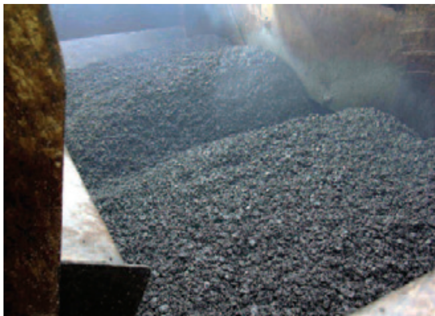
Several thousand tonnes of EME-2 asphalt has been mixed and laid by Lafarge
