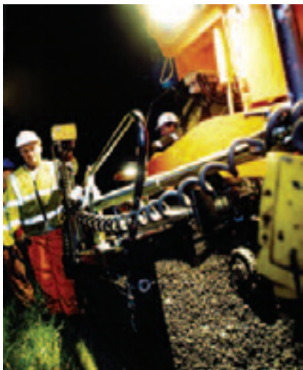
Sasobit was used in a conventional mix to allow the asphalt to be laid at a cooler temperature
