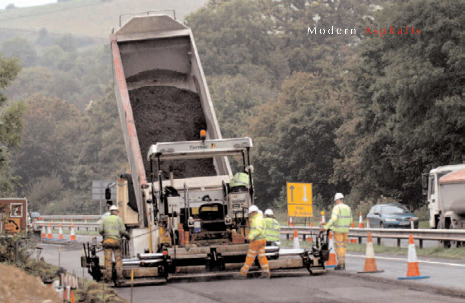
(Above and below) Recycled material is being delivered directly to site for Tarmac to lay and roll the new road surface at a rate of 1,500t per day
