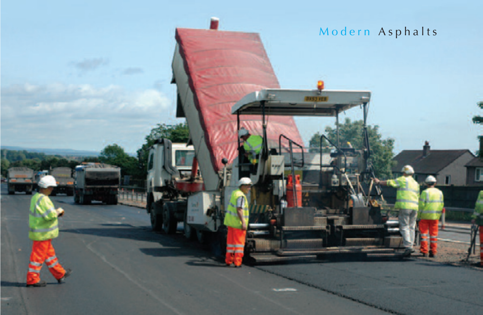
(Above and below) The first surfacing contract to use the draft EME2 specification was carried out by Tarmac on the M876 near Stirling this year
