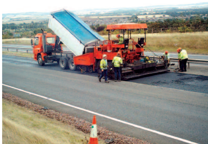
RMC Surfacing is maintaining highways in Scotland and RMC Materials is supplying the asphalt and aggregates
