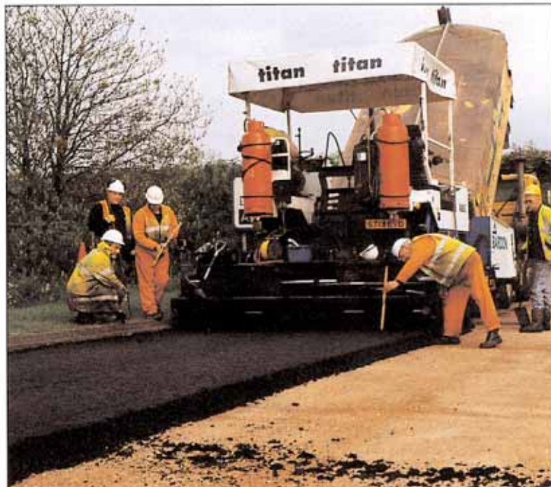
Bardon Surfacing is the BLN JV partner which carries out Area 7 surfacing.
