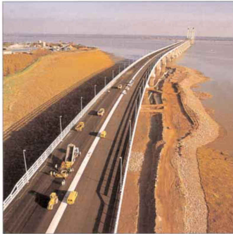
Surfacing works for the second Severn River Crossing were subcontracted to Hanson Construction Projects.
