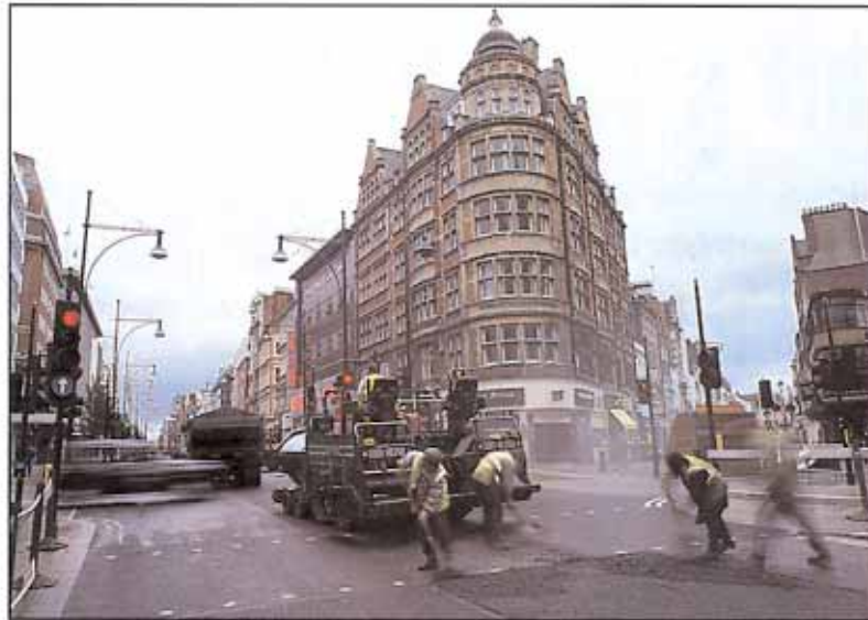
left and far left: Bardon's Hitec being laid in London's Oxford Street
