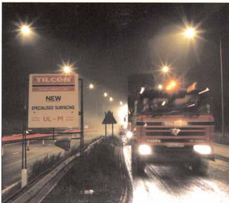
Laying ULM to achieve a durable, quiet surface of high skid resistance
